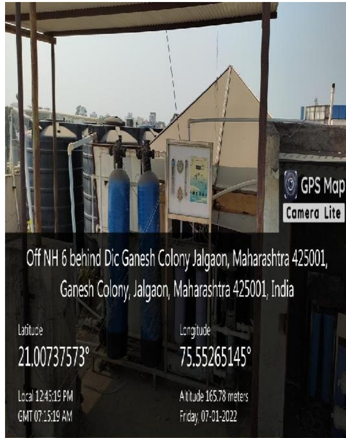
Distribution system in the campus (Centralised RO System)
